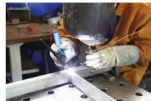
Primary Metal & Installation
